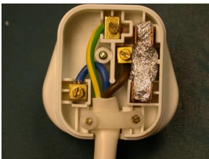
Fuse not being used.
