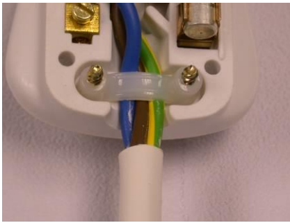
Cable not being gripped.
