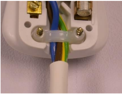
Cable not being gripped.
