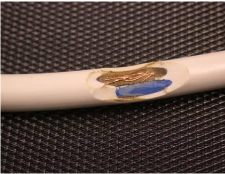
Damage to power cable sheath.
