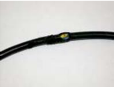
1a Damage to power cable sheath
