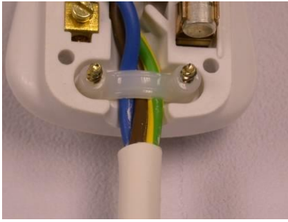
Cable not being gripped.
