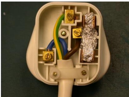
Fuse not being used.
